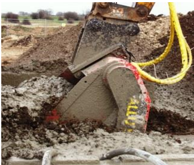
Figure 4 – Mixing of clayey soils with E-Clay (grey coloured slurry) using the specialist processing bucket attachment on a conventional excavator.
