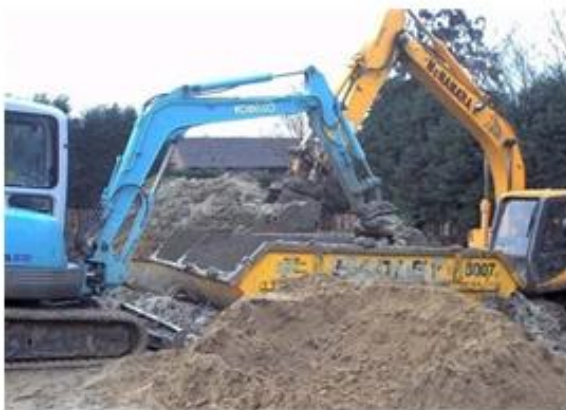
Figure 4 - Set-up of the excavators and skips to mix the contaminated soils with the E-clay® slurry.
