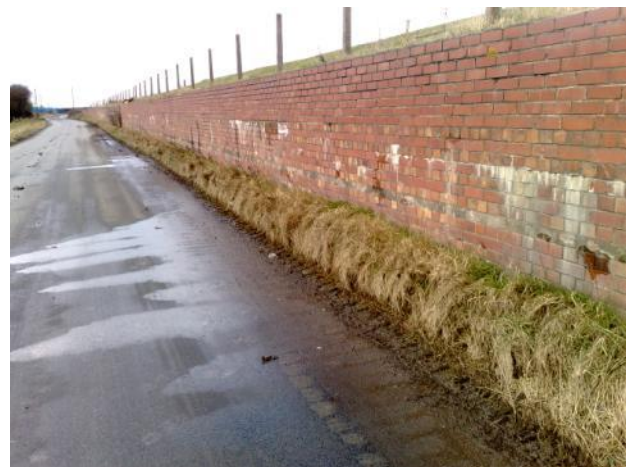
Figure 2 – Evidence of Seepage through Embankment Retaining Wall.
