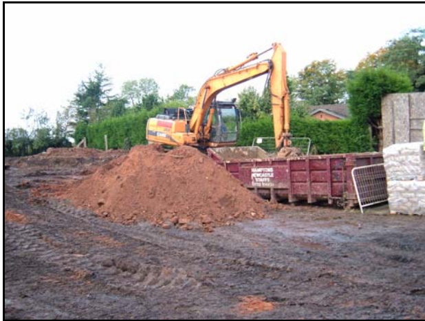
Plate 4 - Set-up of the excavator and skip to mix the contaminated soils with the E-clay ® slurry.
