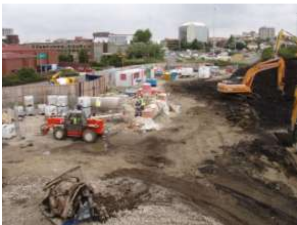
Figure 4 – General site setup with E-Clay slurry manufacture in the centre of the picture.
