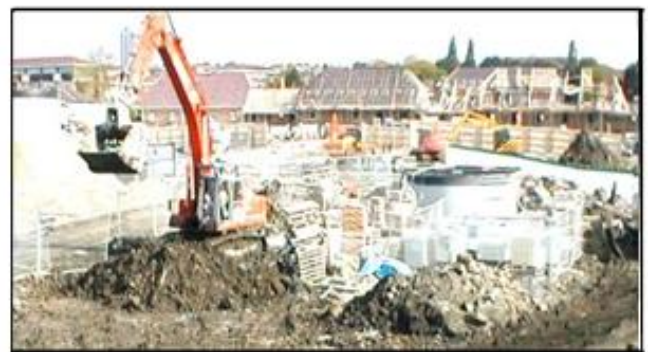
Photo 2 - Treatment of contaminated soils running parallel with Phase 1 of the building program.
