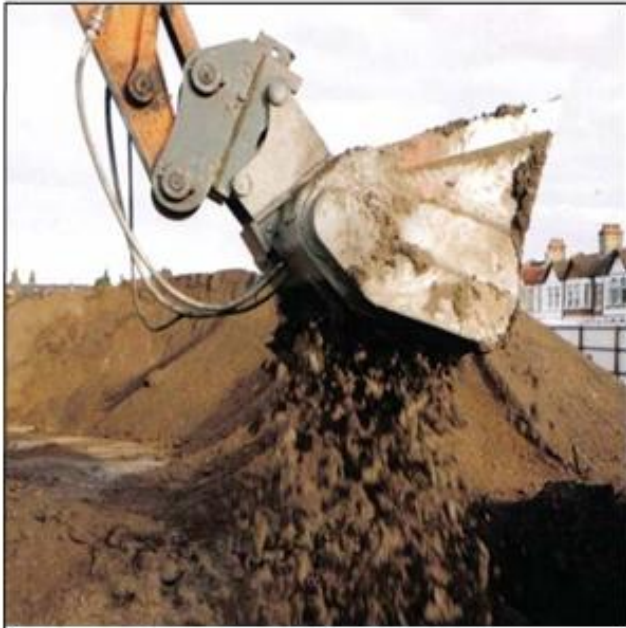
Photo 3 - Mixing of clayey soils with E-clay® slurry using the processing bucket attachment on a conventional 30T excavator.
