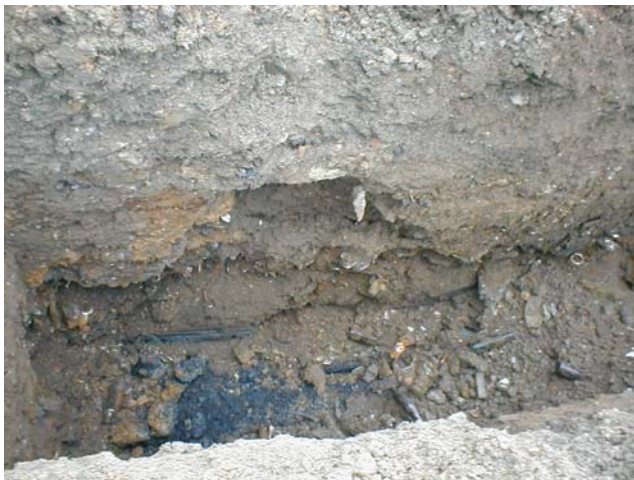
Plate 1: Contaminated soils observed on-site
