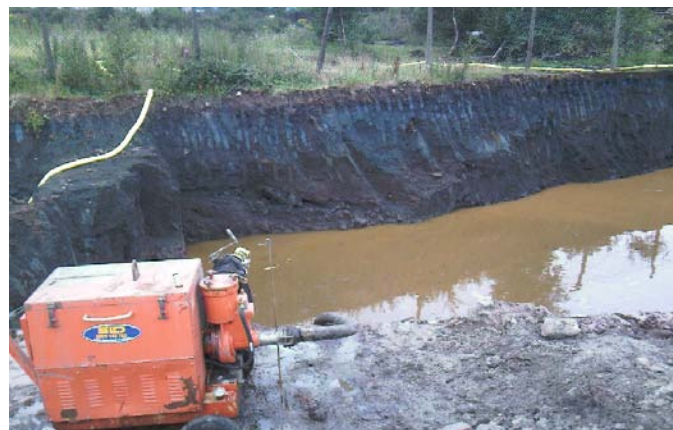
Figure 2 Evidence of contamination associated with a former gas holder.
