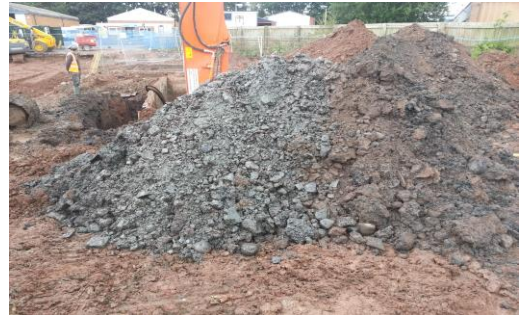
Figure 4 – Hydrocarbon Impacted Soils
