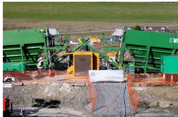
Plate 3 – Fully Automated Batching Plant
