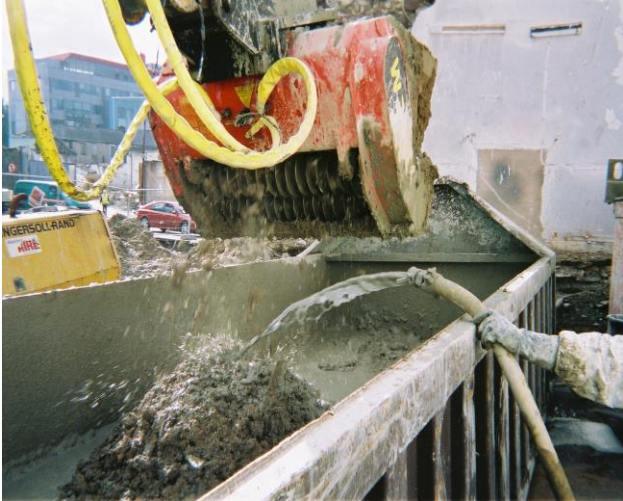
Plate 3 – Mixing of clayey soils with E-clay® slurry using the specialist processing bucket attachment on a conventional excavator.
