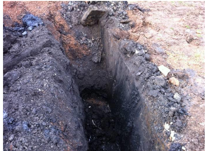
Figure 1 – Typical Gas Works Waste Encountered
